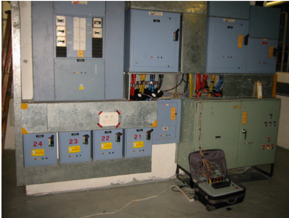
Photo#1 - Site Overview( Switchgears inside Lift Machine Room)
