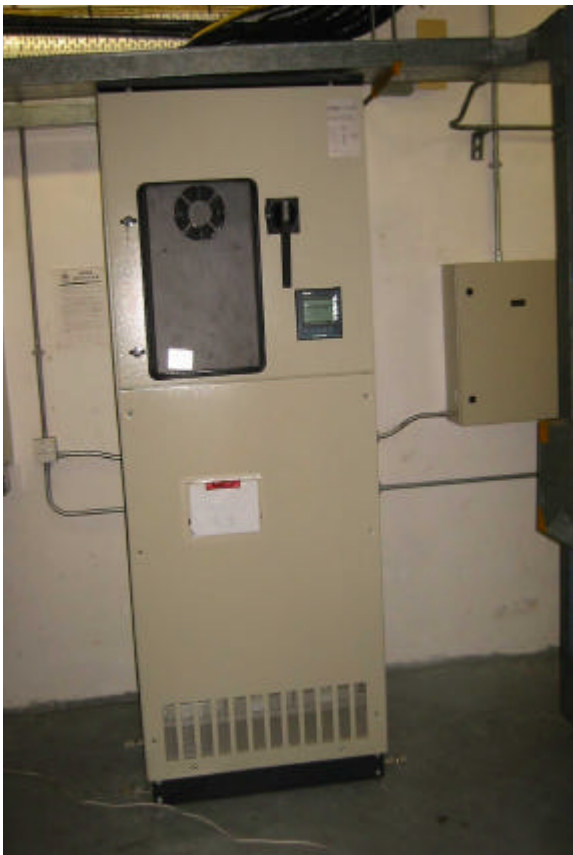
Photo#4 – Real Time Capacitor Bank
