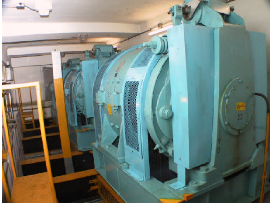
Photo#5 – Lift Motor Drives
